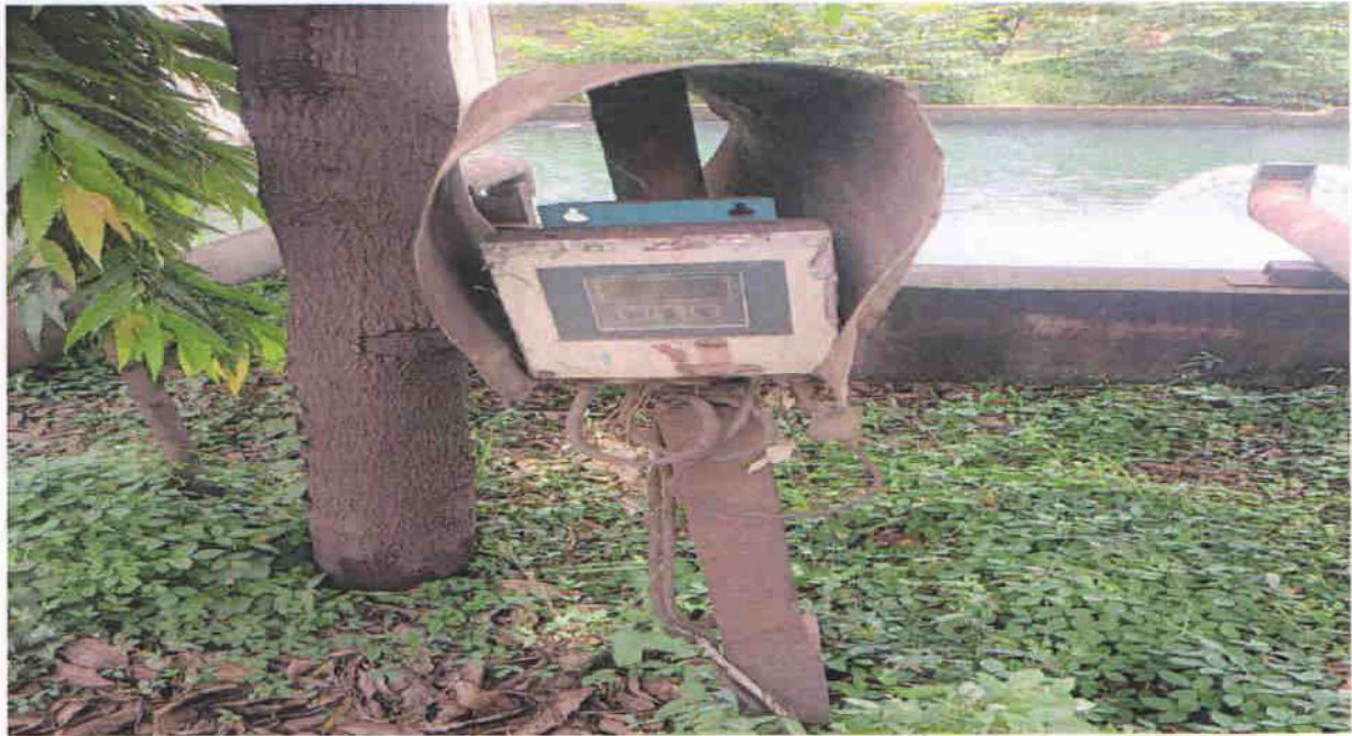
Fig.,- Water meter (Captive Power Plant)
