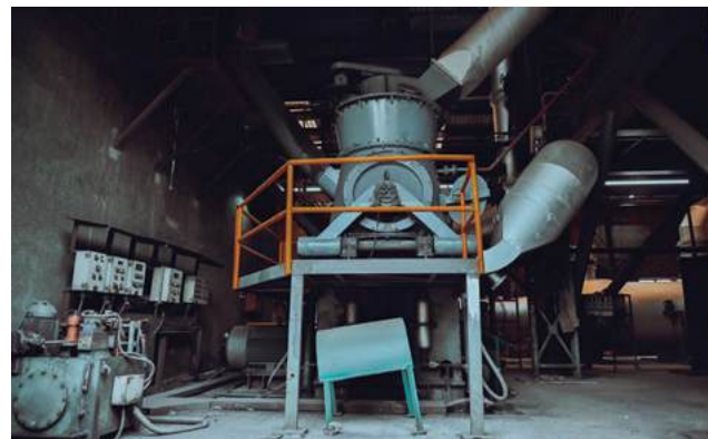
Pulverized Coal Injection (PCI) system to reduce coke consumption and improve furnace efficiency
