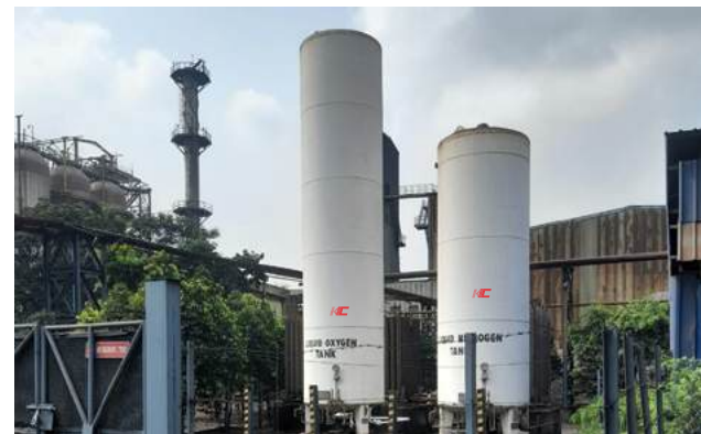
Oxygen and Nitrogen Gas Plants to improve combustion control and process consistency
